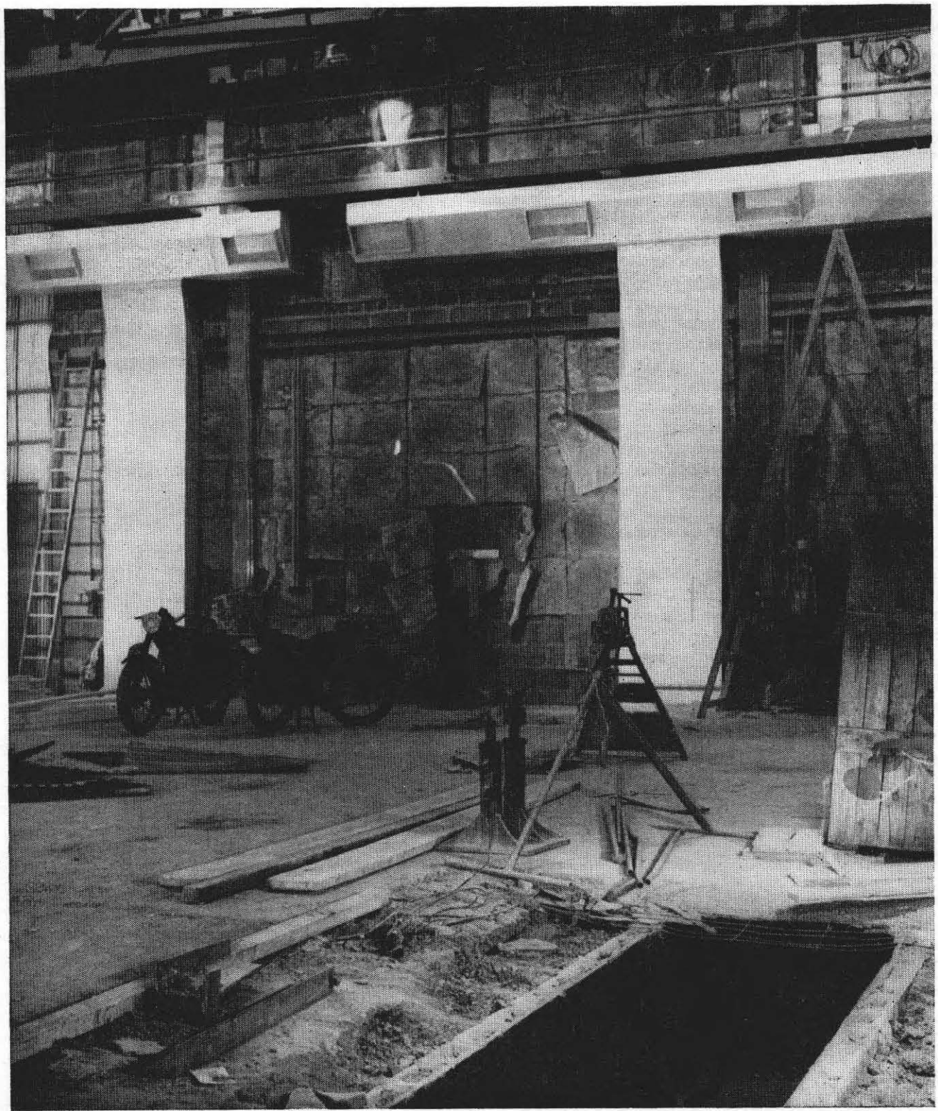
Plate A — Progress photograph showing underground vent ducts and vertical metal risers in Studio 1
